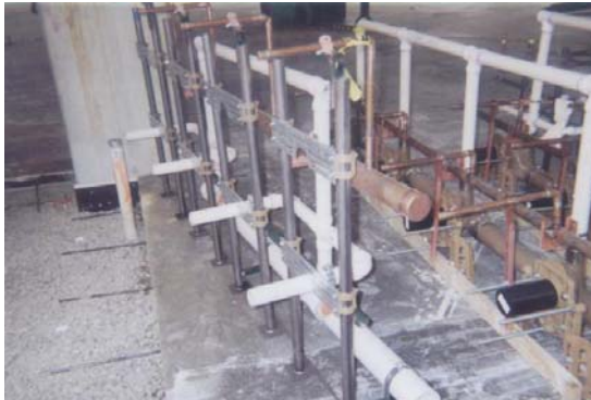
Figure 10A – Concourse toilet Pre-Fab Plbg.
