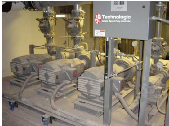
Figure 10 D – Mech Rm. Booster Pumps
