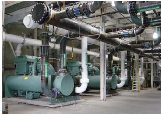
Fig 10B – Chiller Room
